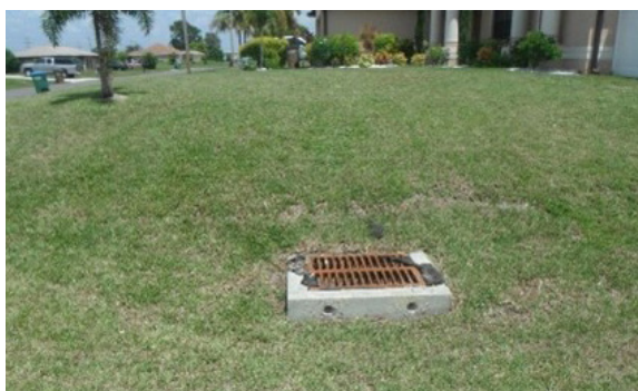
Raised Grate Inlet
