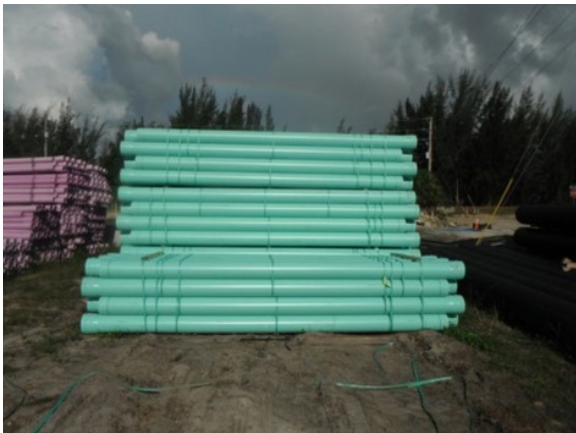
Sewer Pipes (Green Color Pipes)
