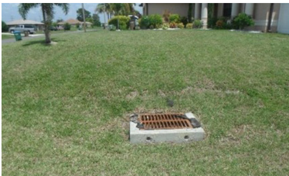
Raised Grate Inlet
